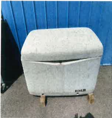
Kohler Generator @ FGM
