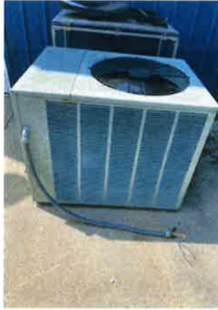
3 Condensing Units @ FGM
